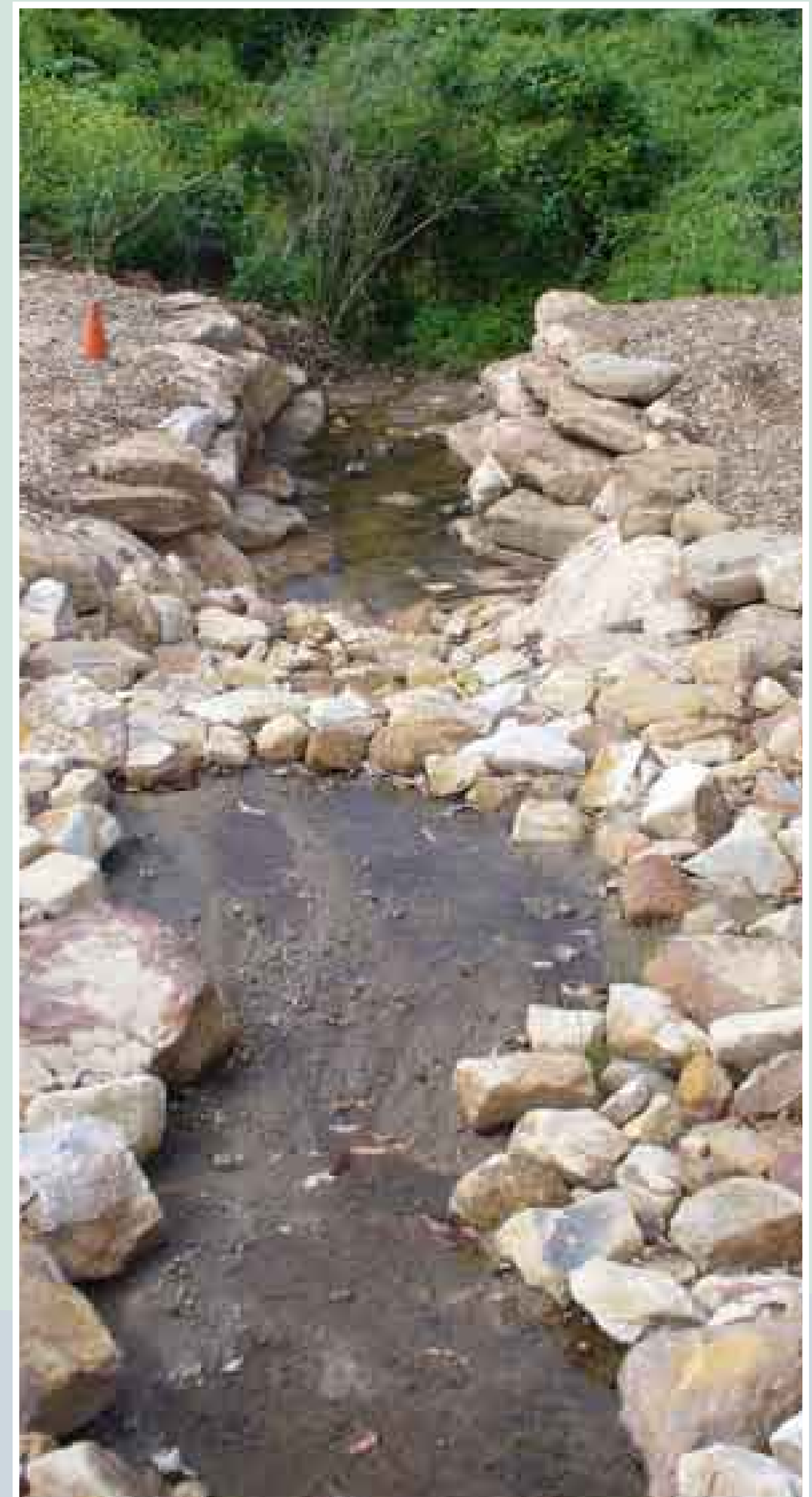
Work has been undertaken to improve the flow of stormwater to Toongabbie Creek
